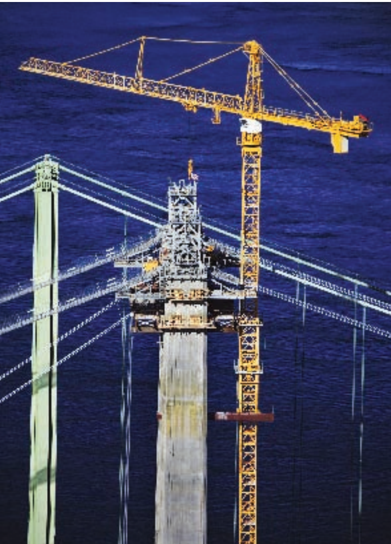
Renovations to structures like the Tacoma Narrows Bridge in Washington State, above, would be virtually impossible without the assistance of tower cranes to do the heavy lifting.
